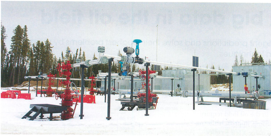
FIGURE 2. The well pads experience freezing temperatures for half of the year, so many well pad functions are contained in heated sheds (background), with one for each wellhead.
